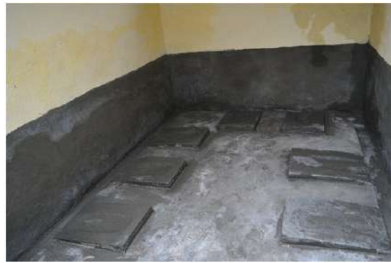
Ladies urinal toilet
